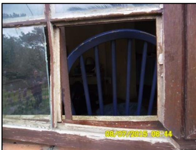
Figure 15: Damaged caused to property by SK6.
